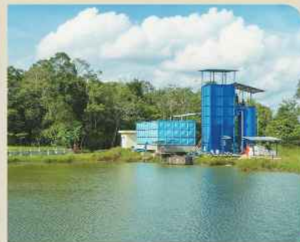
Water Treatment Plant
