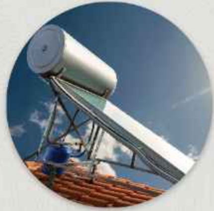
Solar Water Heater
